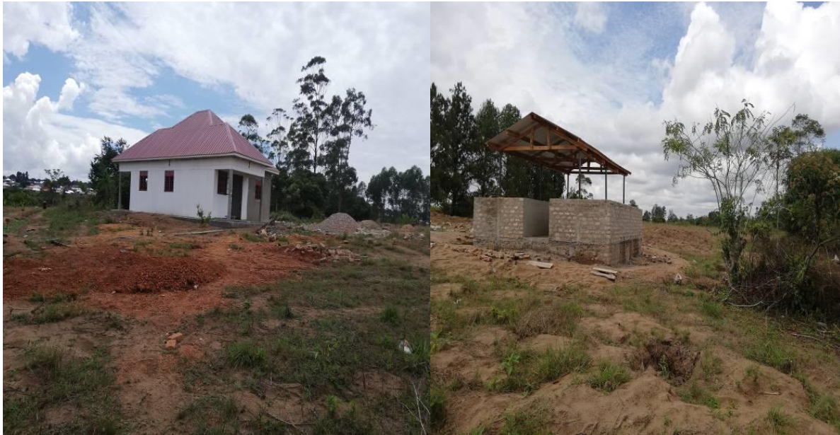
Figure 13: Some of the structures at the organic demonstration farm site under construction
